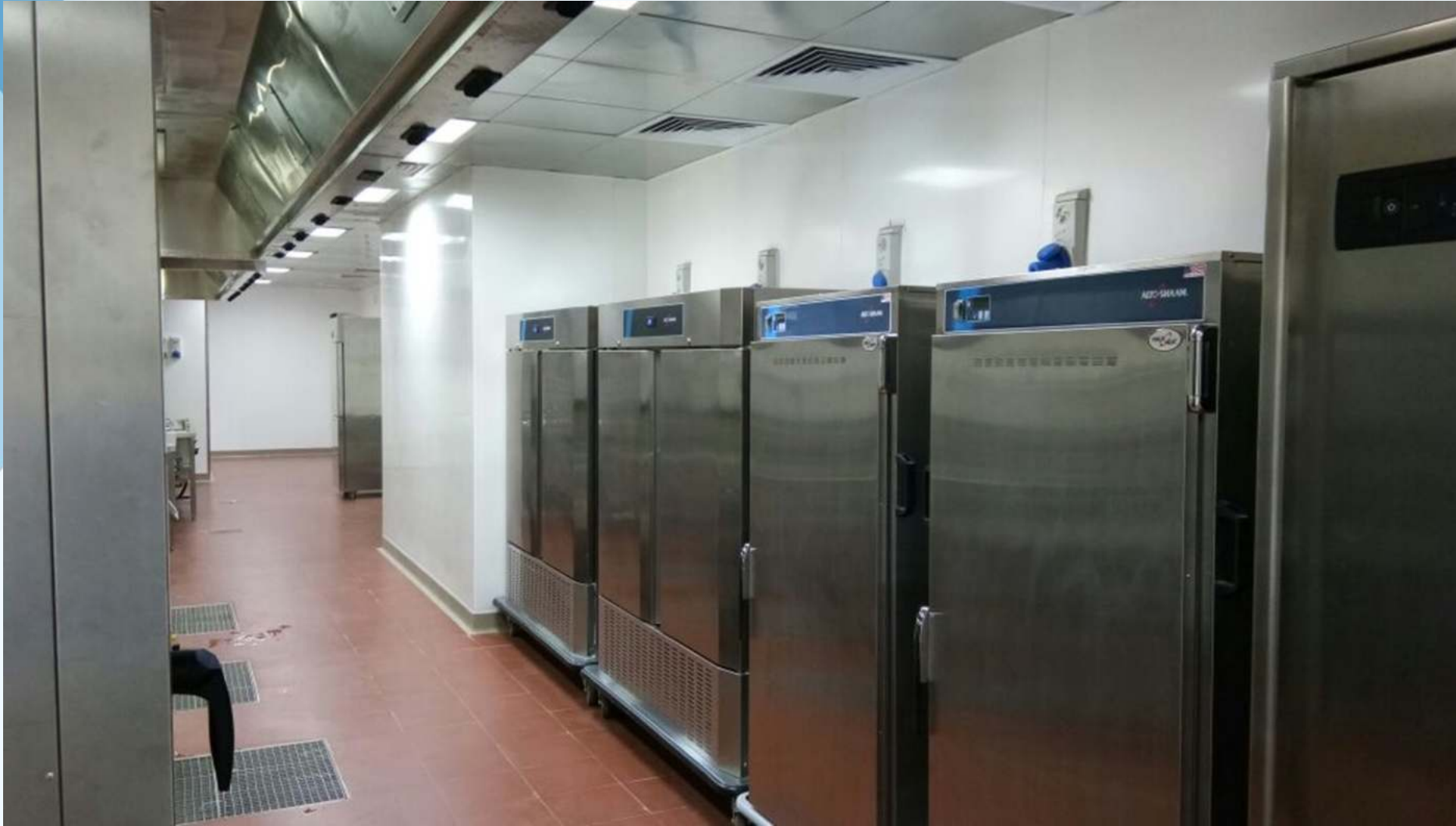
K Ultra - Kitchen Cold Room
